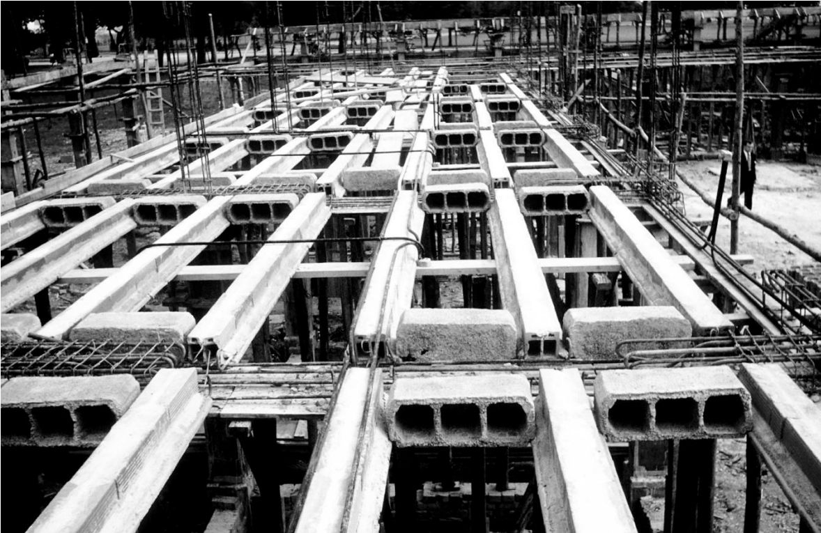
Figura 7. Vista general de la construcción de sistemas de entrepiso en el edificio sede del CINVA. Fuente: Currie, Leonard J. (Leonard James), 1913-1996 (Photographer), "CINVA (Inter-American Housing and Planning Center), Bogotá, Southwest Virginia Digital Archive, accessed June 9, 2022, https://di.lib.vt.edu/items/show/681 .
