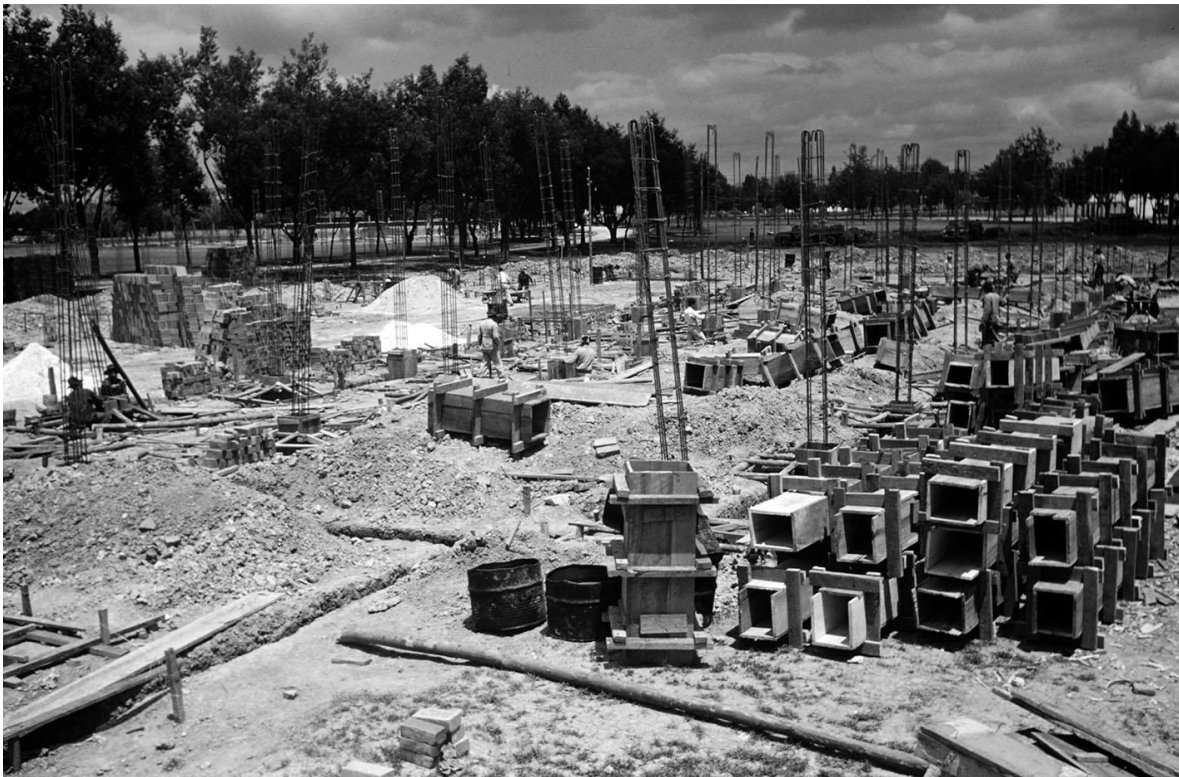
Figura 6. Inicio de la fundición de columnas para la sede del CINVA. Fuente: Currie, Leonard J. (Leonard James), 1913-1996 (Photographer), "CINVA (Inter-American Housing and Planning Center), Bogotá, Southwest Virginia Digital Archive, accessed June 9, 2022, https://di.lib.vt.edu/items/show/681 .
