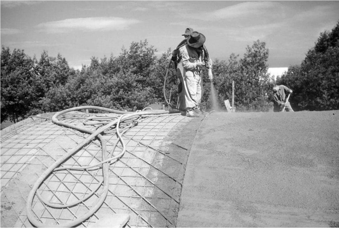
Figura 8. Hormigón proyectado sobre los encofrados de las membranas del edificio CINVA, 1953. Fuente: Currie, Leonard J. (Leonard James), 1913-1996 (Photographer), "CINVA (Inter-American Housing and Planning Center), Bogotá, Southwest Virginia Digital Archive, accessed June 9, 2022, https://di.lib.vt.edu/items/show/673 .
