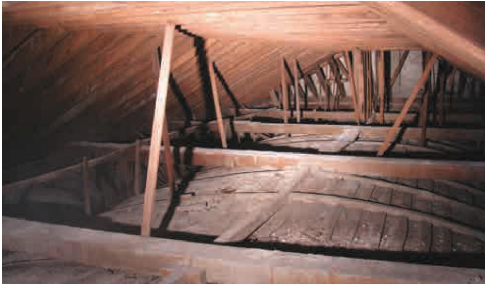
Figure 47. Typical Colonial Roof structure. Cathedral of Santiago de Cuba, Cuba Source: Elena Perria, 2010.
